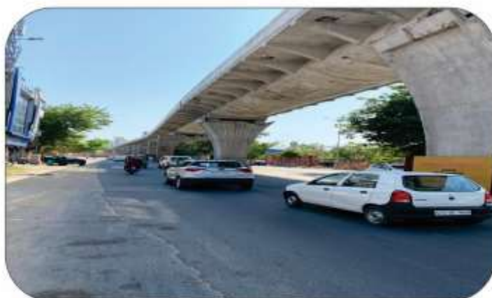
Construction of Elevated Road from Sodala Tri-junction to LIC Office near Ambedkar Circle, Jaipur by JDA [Estimated Cost – Rs. 225 Cr; Loan Sanctioned – Rs. 169 Cr.]
