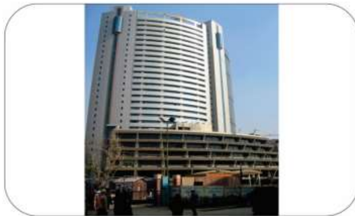
Construction of MCD Office and Civic Centre, New Delhi [Estimated Cost – Rs. 410.56 Cr; Loan Sanctioned – Rs. 250 Cr.]
